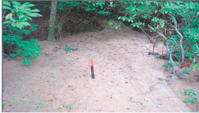
Photo 4: High degree of sedimentation along UWC-10L-2R-1R-B in the Stonehouse development along the golf
