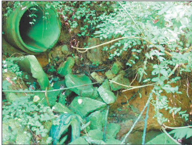
Photo 6: Eroded outfall located at the head of FRS-14R-4L-A in Mirror Lakes Estates residential development.
