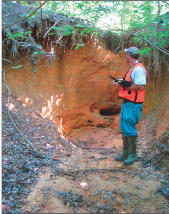
Photo 3: Headcut located within the Stonehouse Commercial Park at upstream end of SAR UWC-3R-A.
