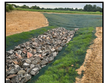
Below: The finished product of a different head cut that had impacted a crop field. This rock lined chute reduces stormwater energy and releases the flow into the natural channel down slope.
