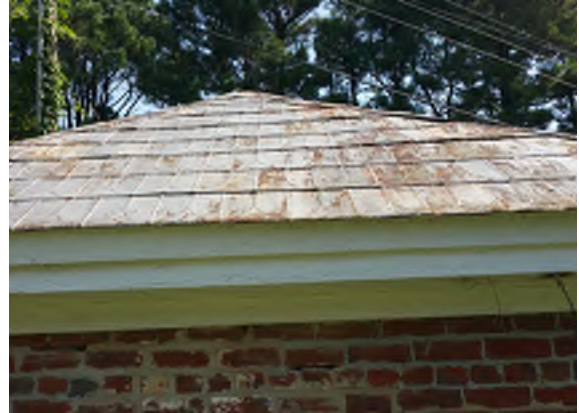
Smokehouse roof deterioration
