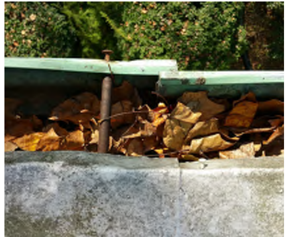
Gutters at porch roof needing repair
