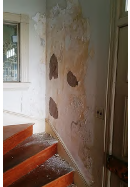
Plaster damage from moisture issues
