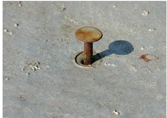
Nail in porch roof repair area
