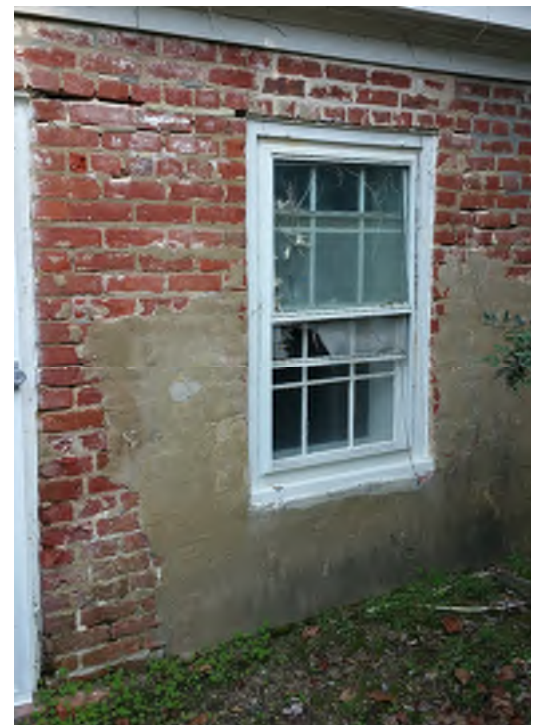
Brick Issues at Servant Quarters
