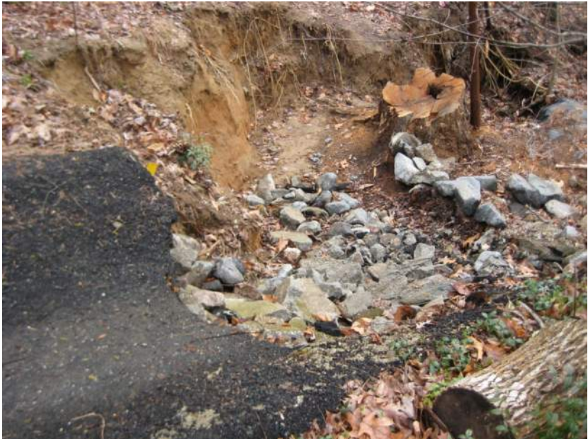
Broken, Eroding Paved Ditches
