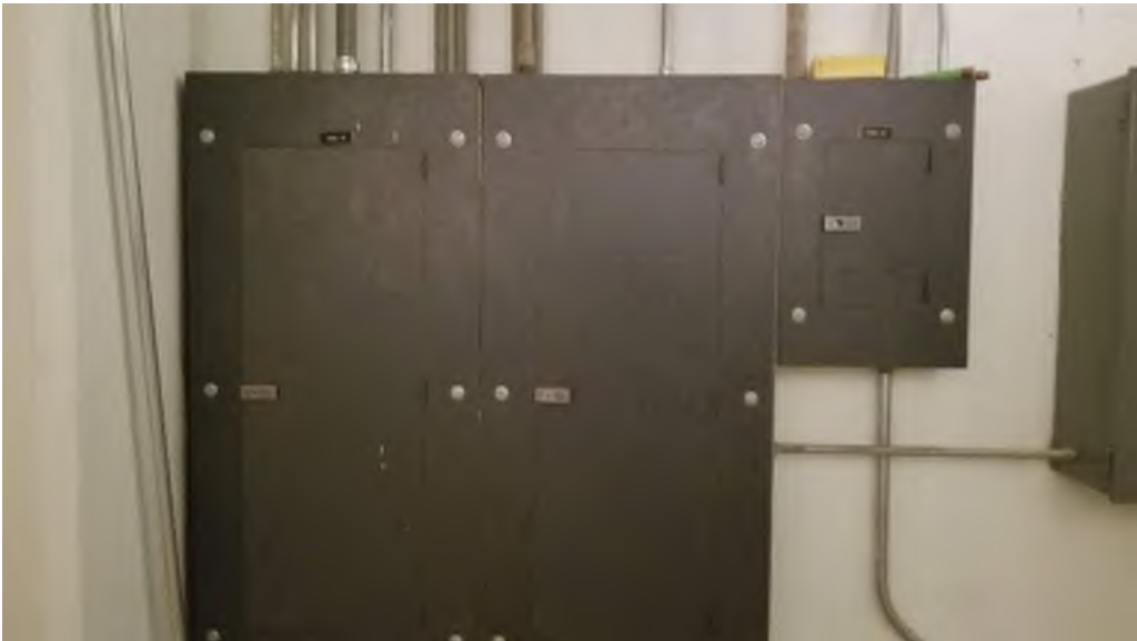
Panelboards in Original Section of the Building
