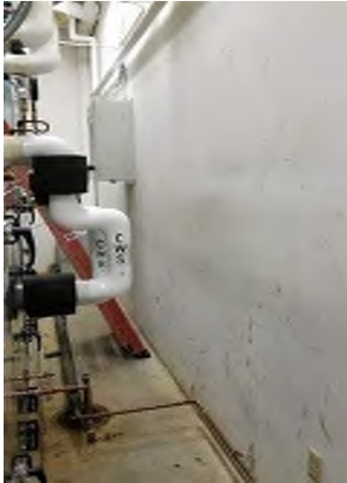
Controls and Disconnect Switch Located Behind Air Handling Unit (Code Violation)
