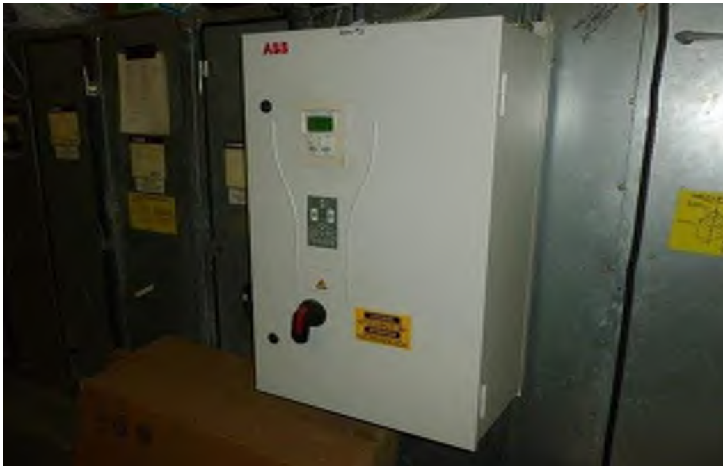
AHU-3 with Variable Frequency Drive Manufacturer: Trane (1997), ABB Supply Fan Frequency Drive (2006)
