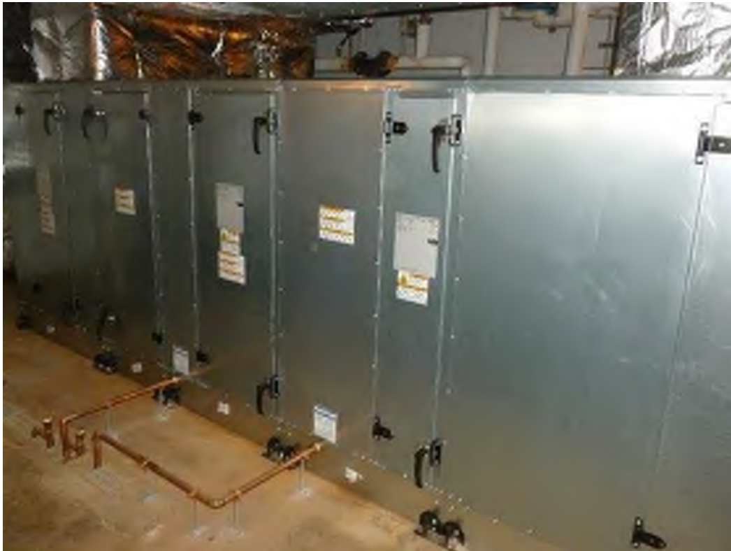
AHU-2 with VFD Manufacturer: Trane (2017) Model No.: CSAA030UAL00
