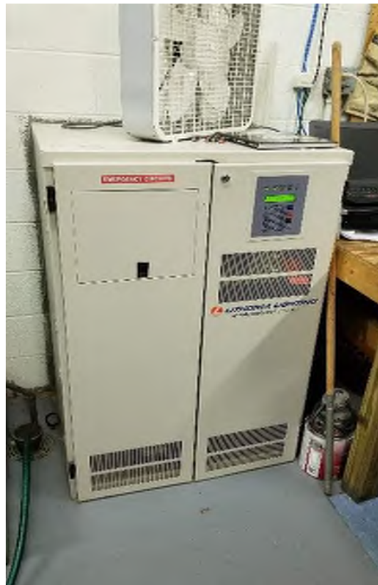
Emergency Battery Backup System (Installed in 2009)
