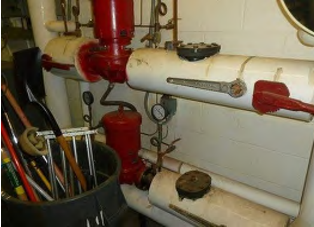
Inline Primary and Secondary Heating Hot Water Pumps Manufacturer: Bell and Gossett
