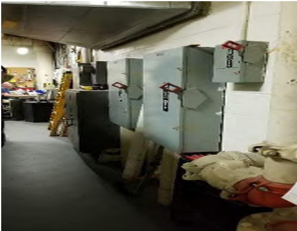
Two 400A Main Service Disconnect Switches Fed from Power Company's CT Cabinet
