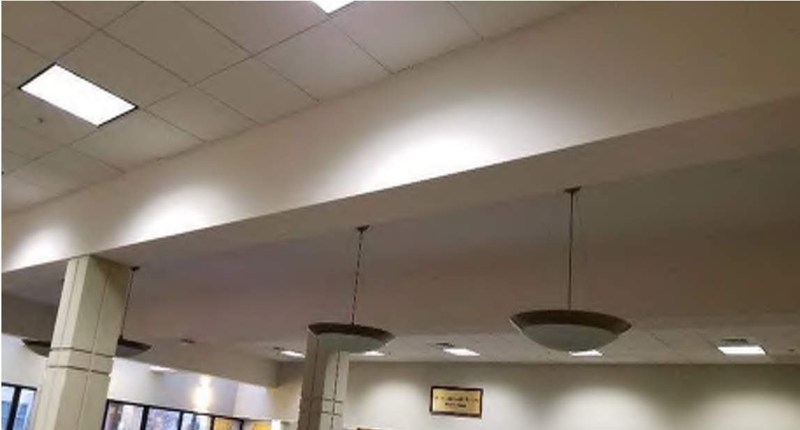
Lighting in Computer Station Area
