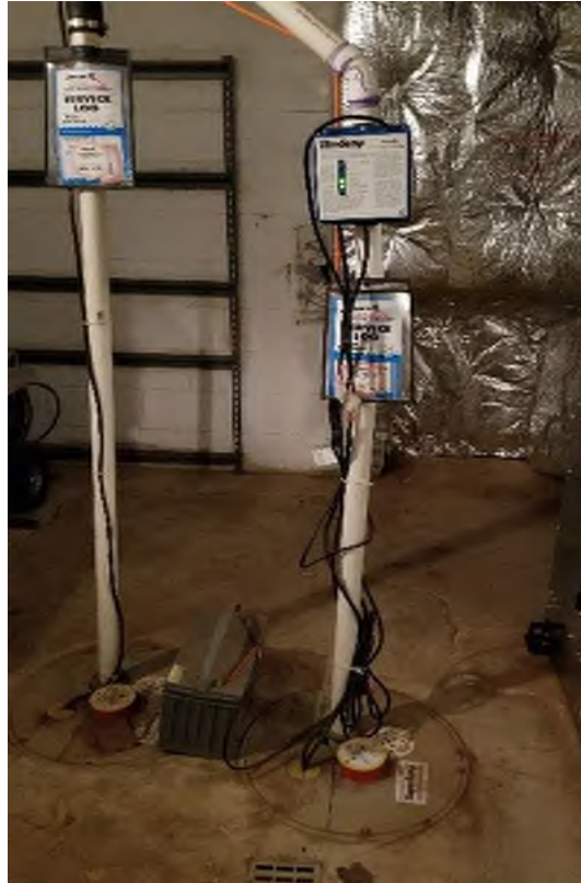
Sump Pump with Battery Backup
