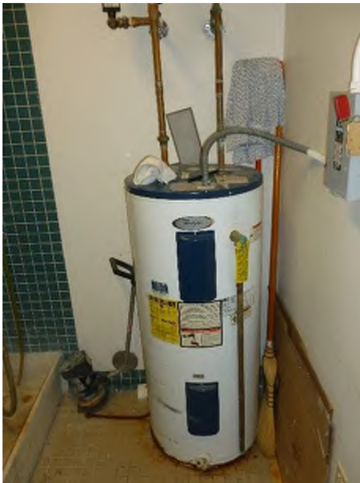
40 Gallon Electric Water Heater (Lobby 2) Manufacturer: Whirlpool US Craftmaster (1999) Model No.: E2F40RD045V
