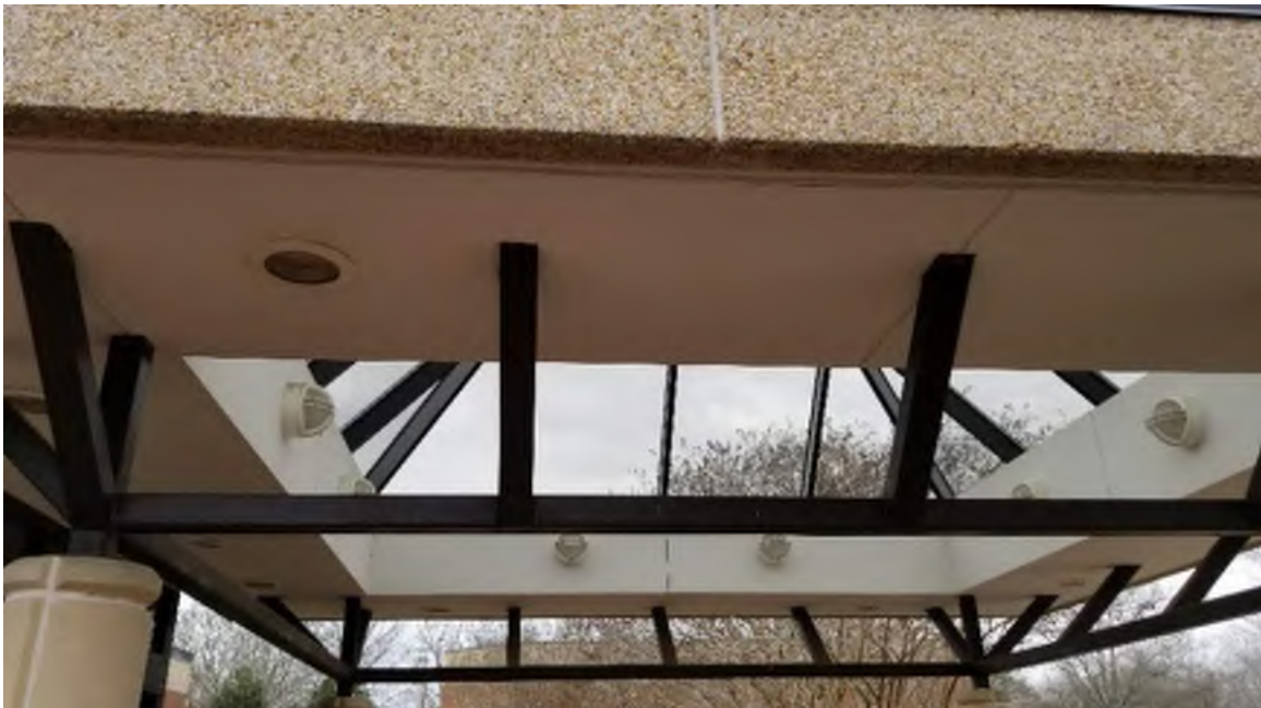
Exterior Canopy Lighting
