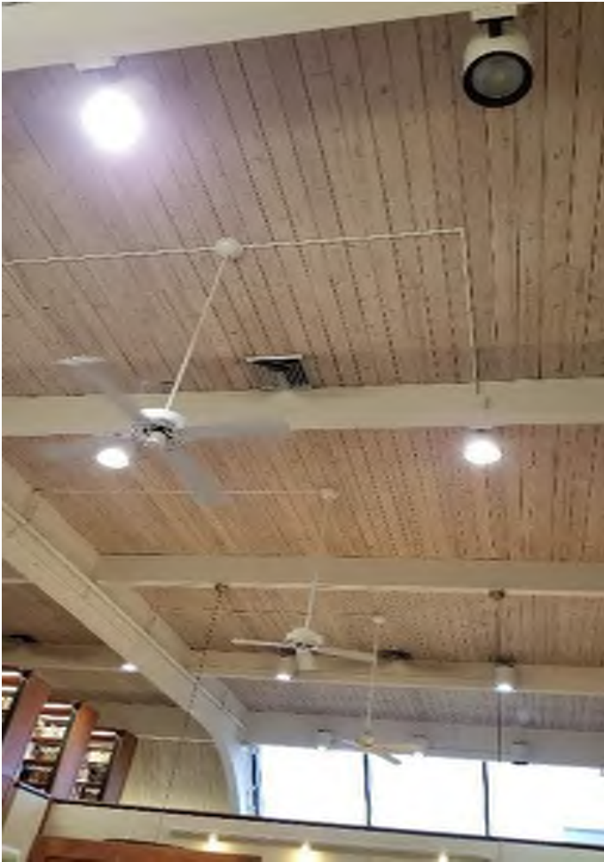
Library Area Lighting
