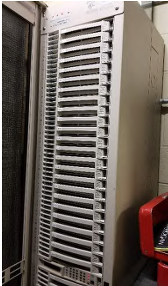
Theater Lighting Control Panel
