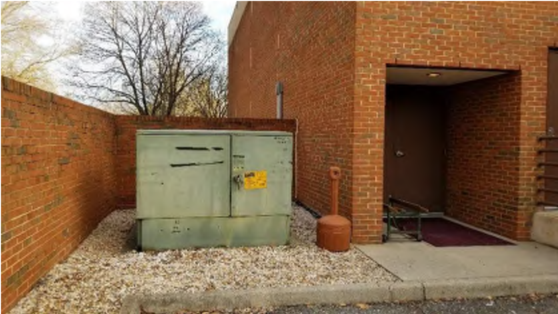
Power Company's Pad Mounted Transformer
