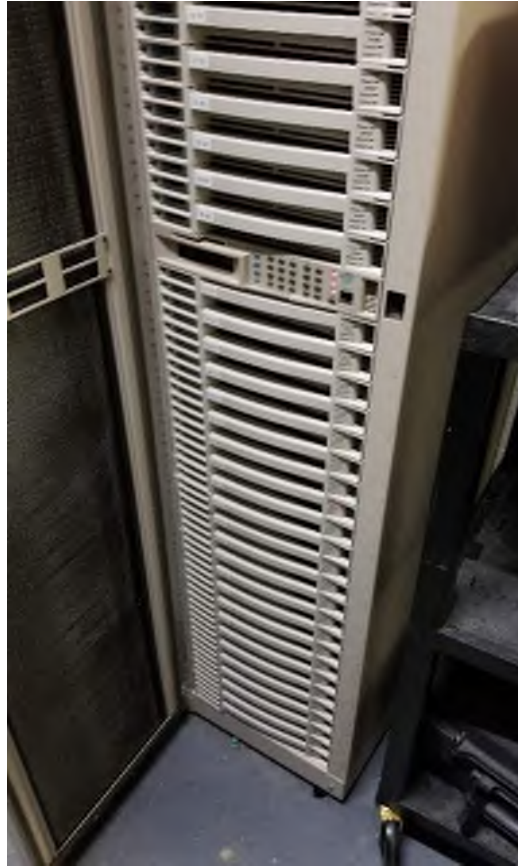
Theater Lighting Control Panel
