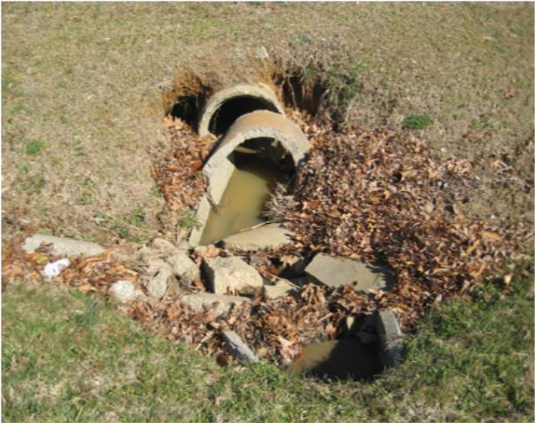
Aging, Failing Storm Drains
