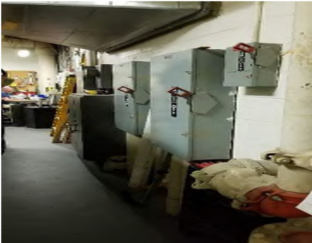
Two 400A Main Service Disconnect Switches Fed from Power Company's CT Cabinet
