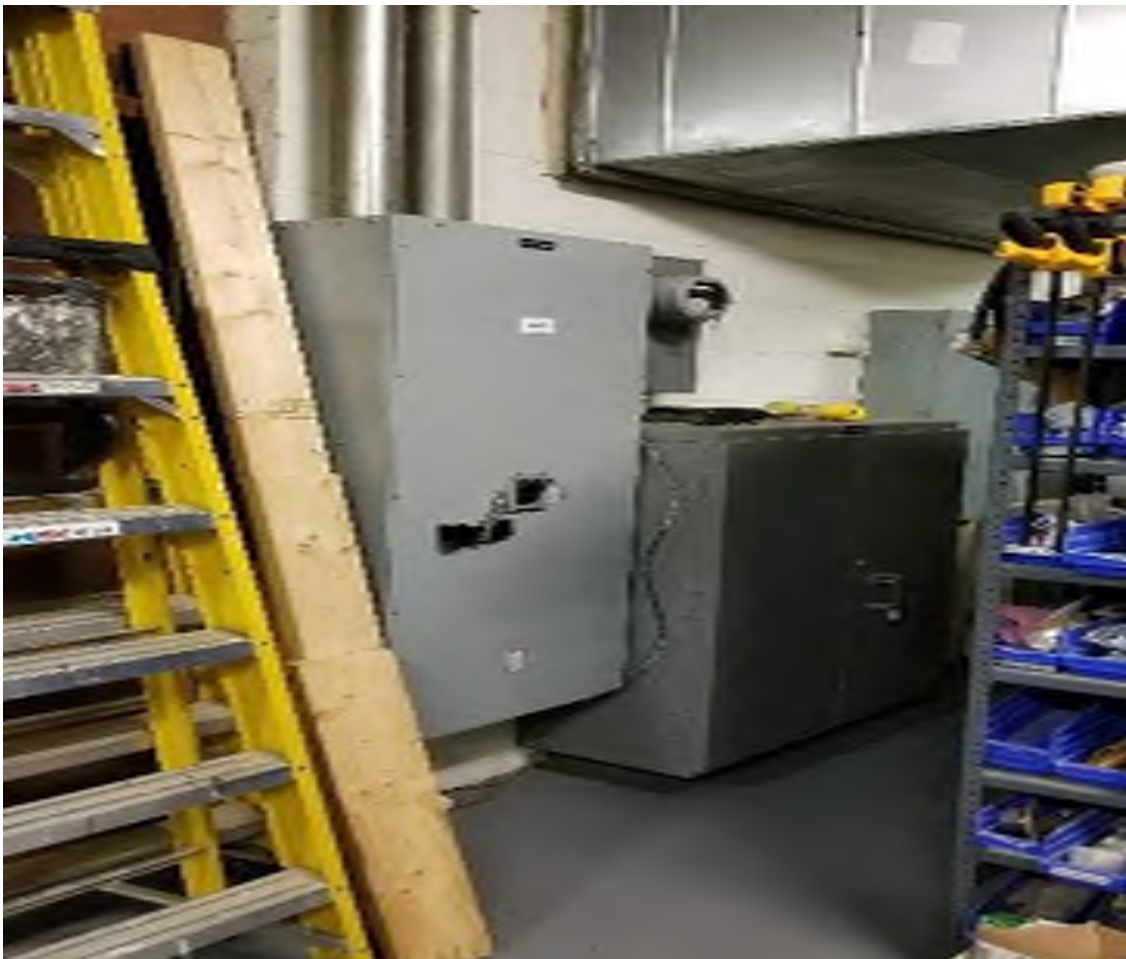
800A Enclosed Circuit Breaker And Power Company's CT Cabinet
