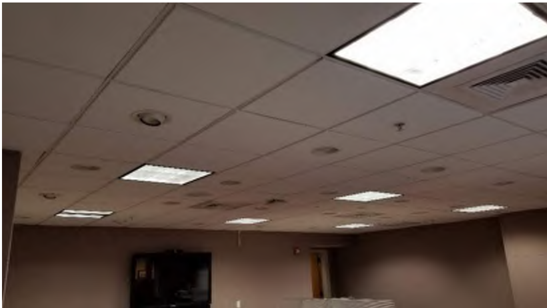
Fluorescent and Incandescent Fixtures in Schell Room
