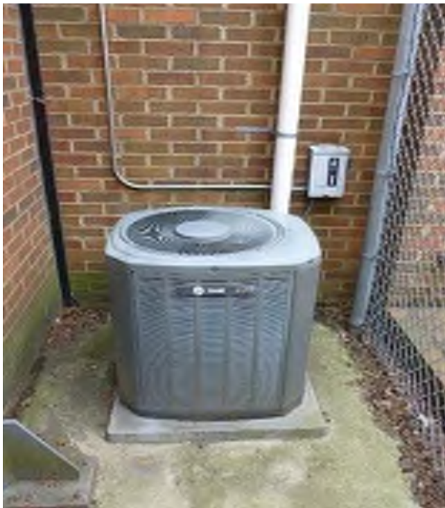
Ducted Split System Heat Pump (Outdoor Unit) Manufacturer: Trane (2003) Model: 2TWR2024A1000AB
