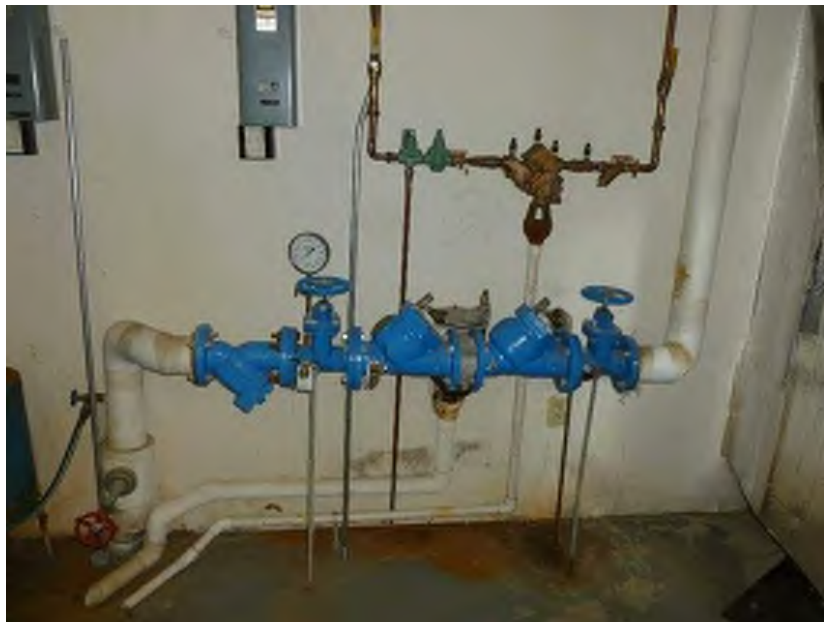
2-1/2" Domestic Water Reduced Pressure Type Backflow Preventer 3/4" Chilled Water Make-Up Reduced Pressure Type Backflow Preventer
