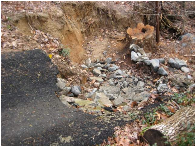
Broken, Eroding Paved Ditches
