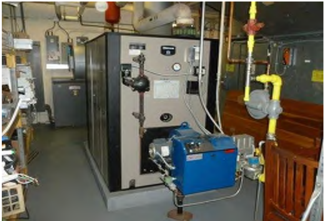
Oil/Natural Gas Fired Boiler (2009) with Conversion to Natural Gas (2013) Manufacturer: Weil-McLain Model No.: 788
