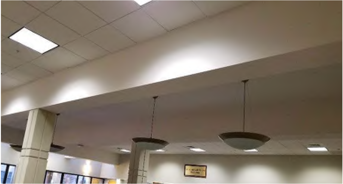
Lighting in Computer Station Area
