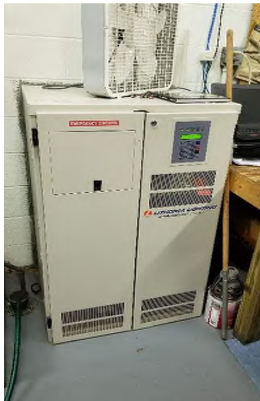
Emergency Battery Backup System (Installed in 2009)
