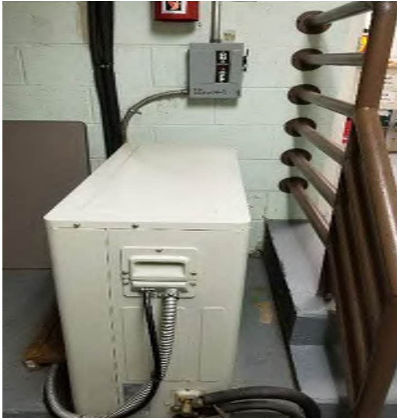
Disconnect Switch for Mini-Split is Installed Behind Unit (Code Violation)
