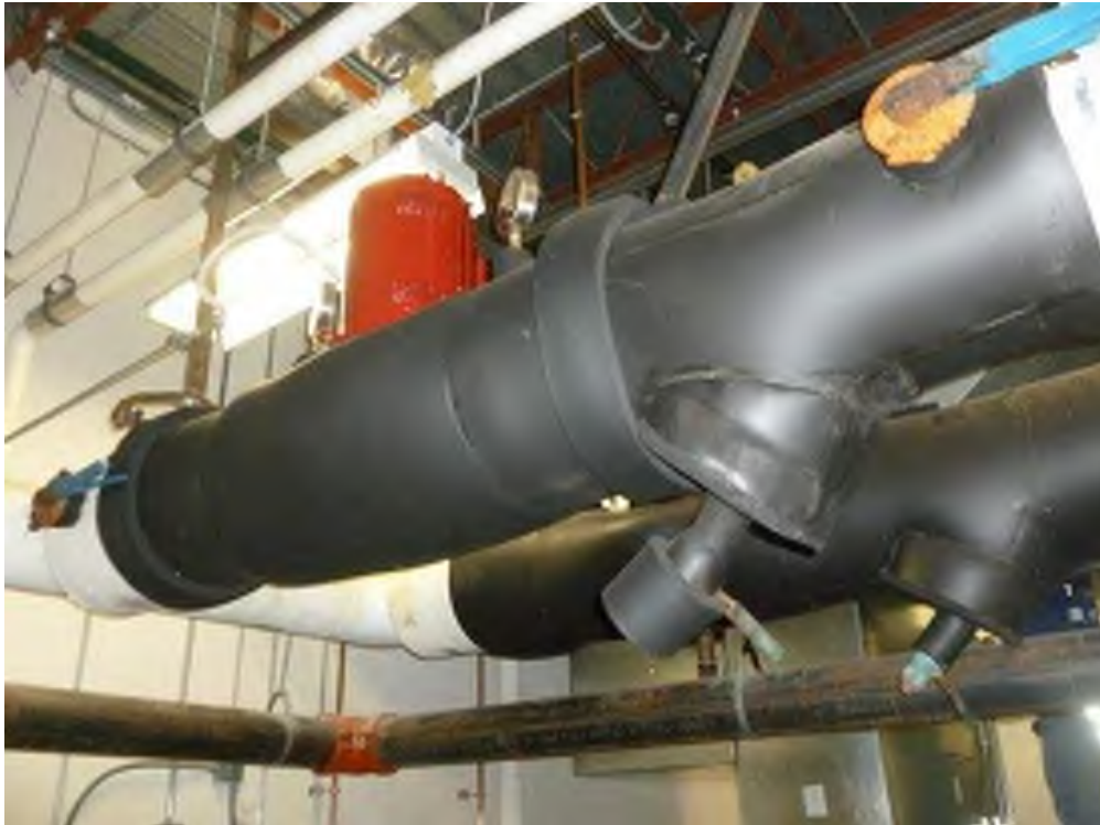
Inline Primary and Secondary Chilled Water Pumps Manufacturer: Bell & Gossett
