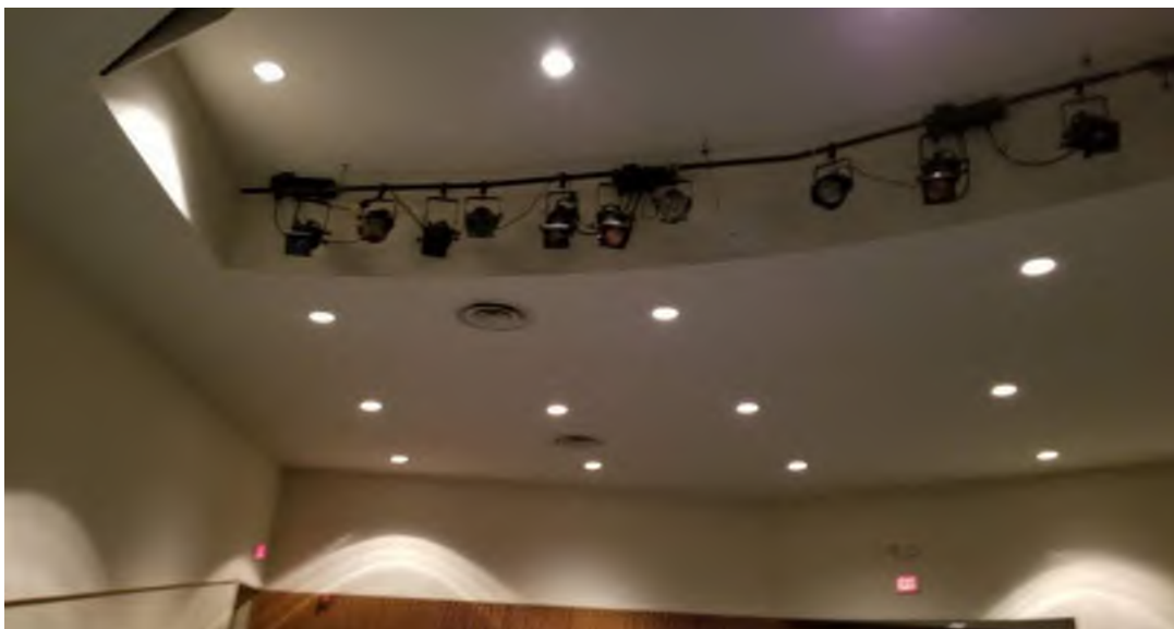
Theater Lighting Compact Fluorescent Downlights and Specialized Theater Spot Lights
