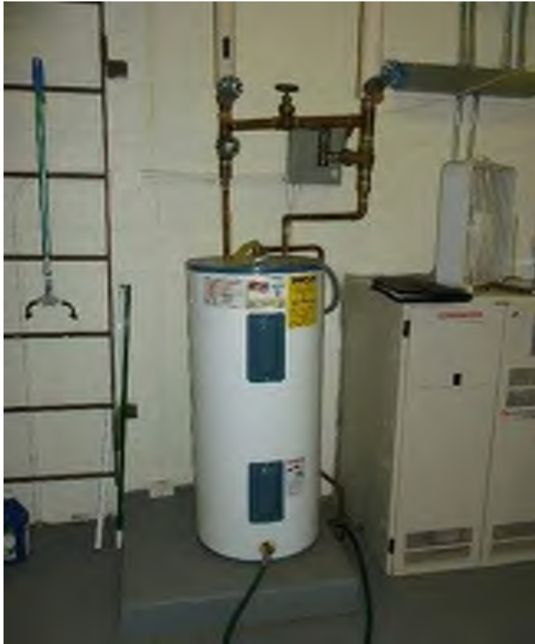
40 Gallon Electric Water Heater (Lobby 1) Manufacturer: RUUD Model No.: PE40-2D
