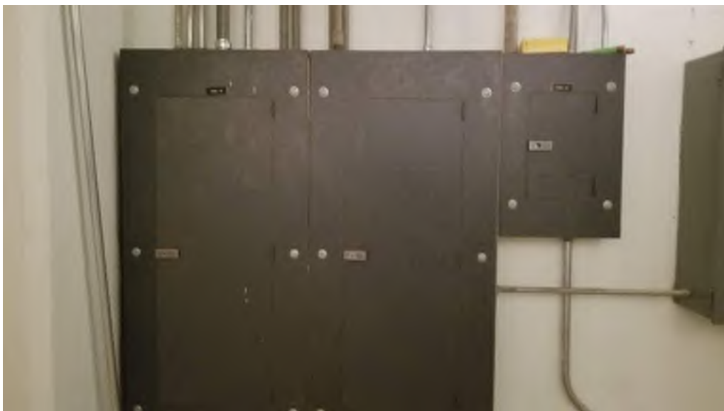
Panelboards in Original Section of the Building
