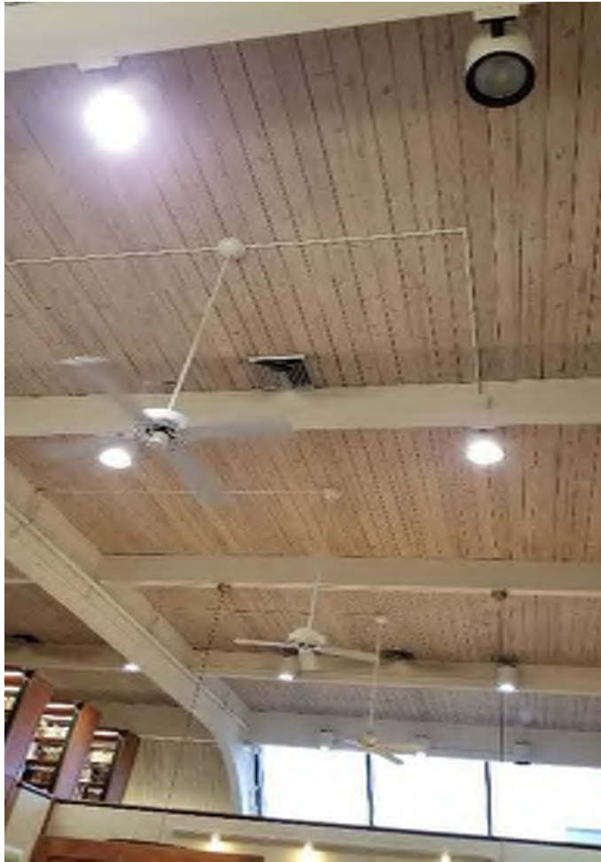
Library Area Lighting
