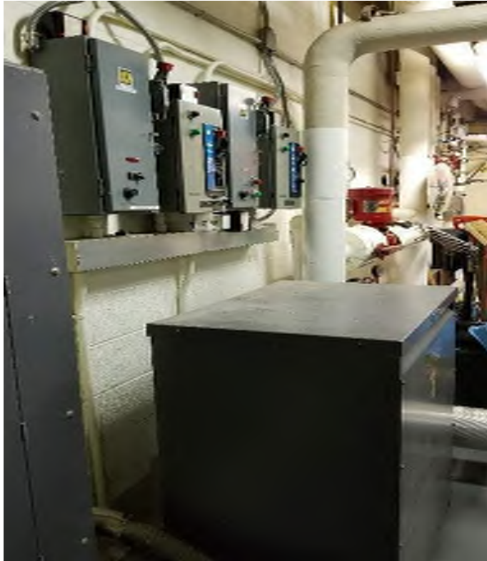
Bank of Disconnect Switches Installed behind Dry Type Transformer (Code Violation)
