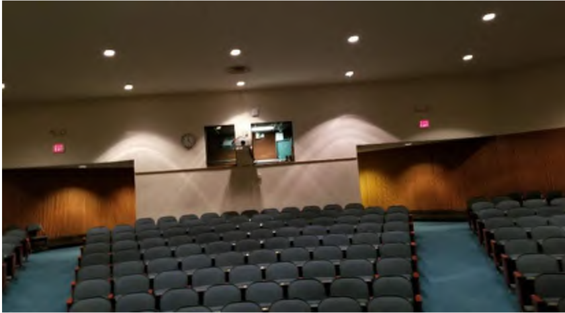
Theater Lighting and Control Room
