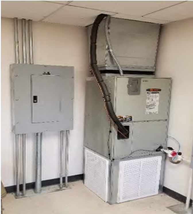
Panelboards in Renovated Area
