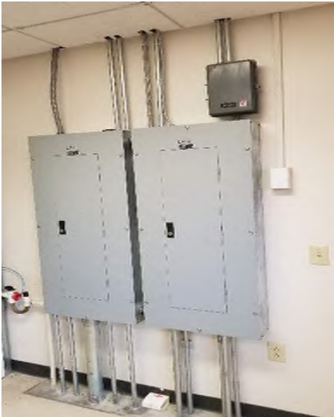
Panelboards in Renovated Area
