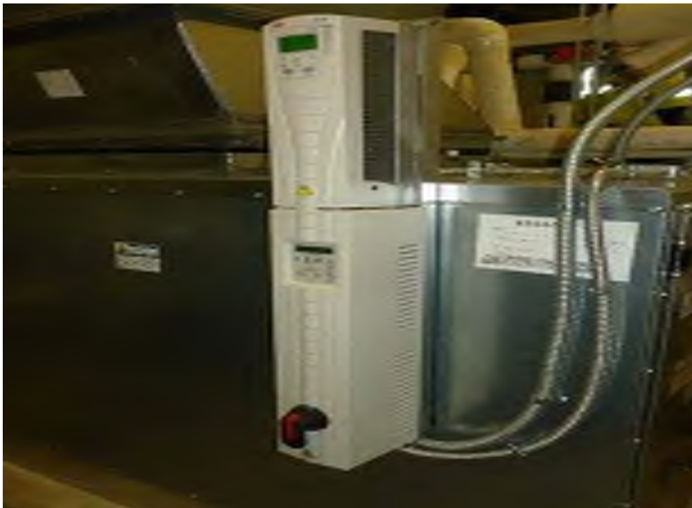
AHU-1 with Variable Frequency Drive Manufacturer: Trane (2018) Model No.: CSAA021UAL00
