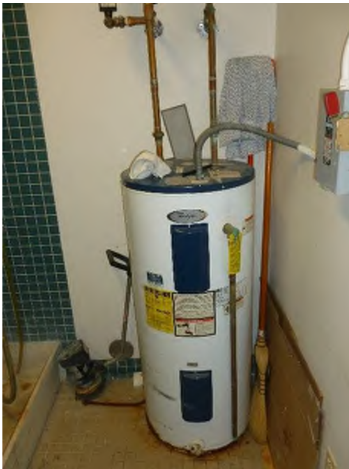
40 Gallon Electric Water Heater (Lobby 2) Manufacturer: Whirlpool US Craftmaster (1999) Model No.: E2F40RD045V
